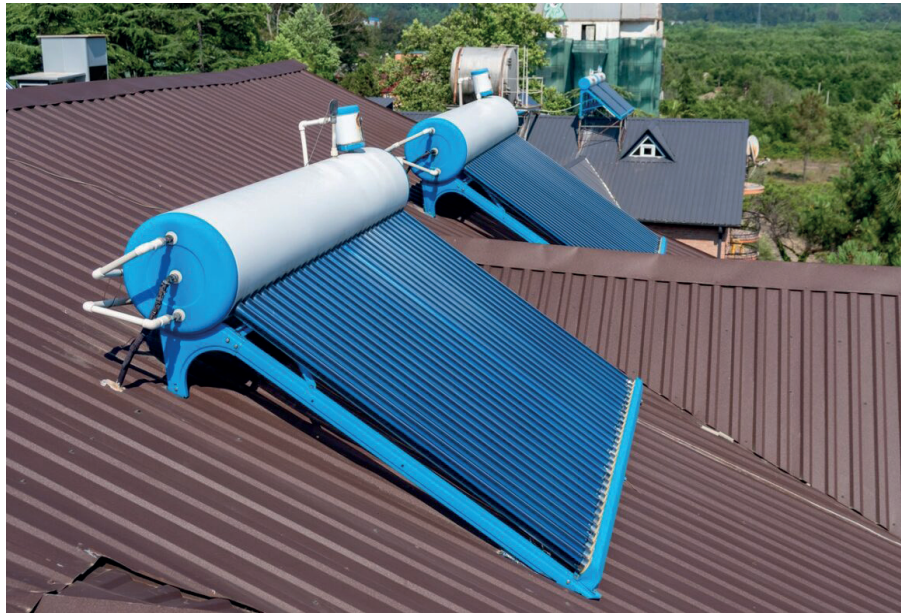
Figure 3: Solar water heaters on rooftops
